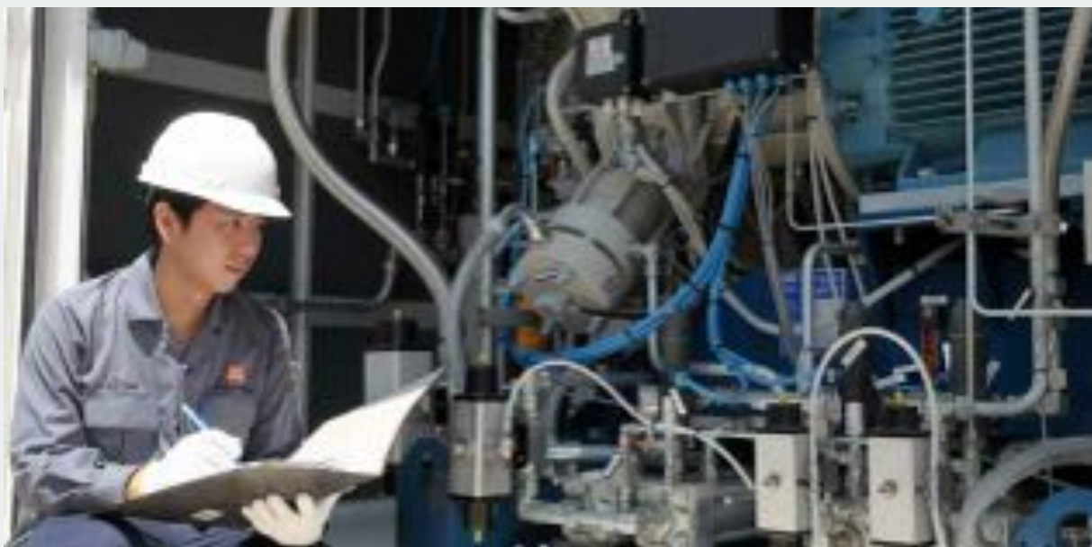
Sime Darby Offshore Engineering (SDOE) was the lead technology provider for the first biogas plant in Malaysia to produce Bio-CNG.
