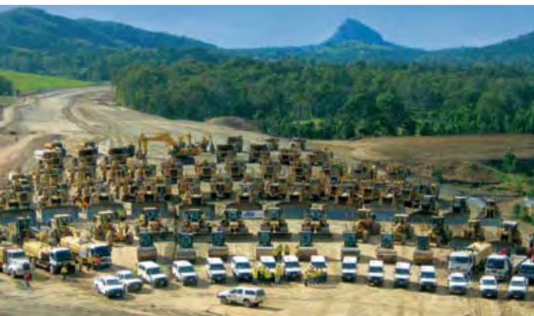
Rows of Caterpillar equipment used for the Bruce Highway upgrading project in Queensland, Australia
