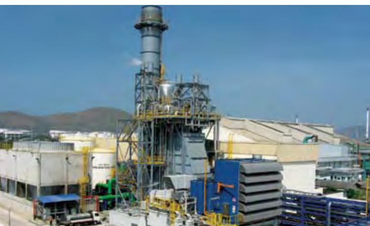
The newly completed Sime Darby LCP Power Co Ltd (SLP) power plant
